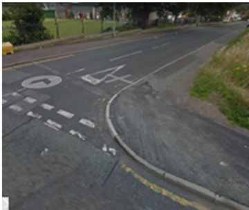
- Highfield Road and Rockcliffe Street junction showing tyre tracks across the resurfaced pavement.
